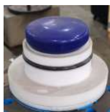
Outside flange & Nozzle neck damaged 外法蘭及頸部破損
